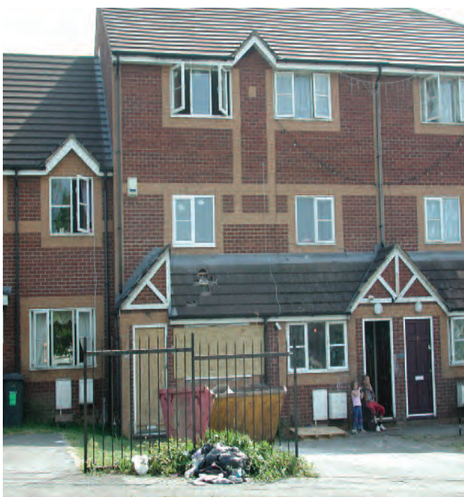
Maisonettes on Gainsborough Square in need of good housing management and maintenance
